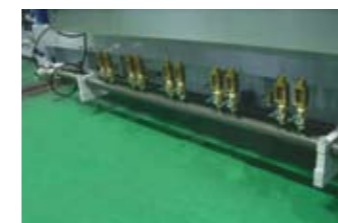
Mold cooling water closed circuit (bed installing type)
